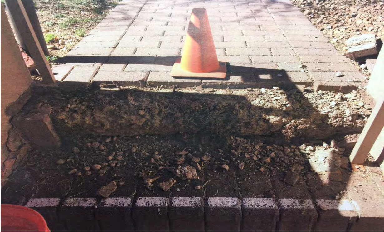
3. Stair and walkway weather and use deterioration
