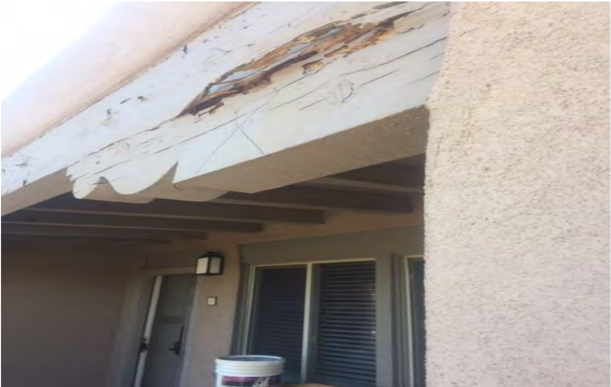
4. Header and Corbel water intrusion damage
