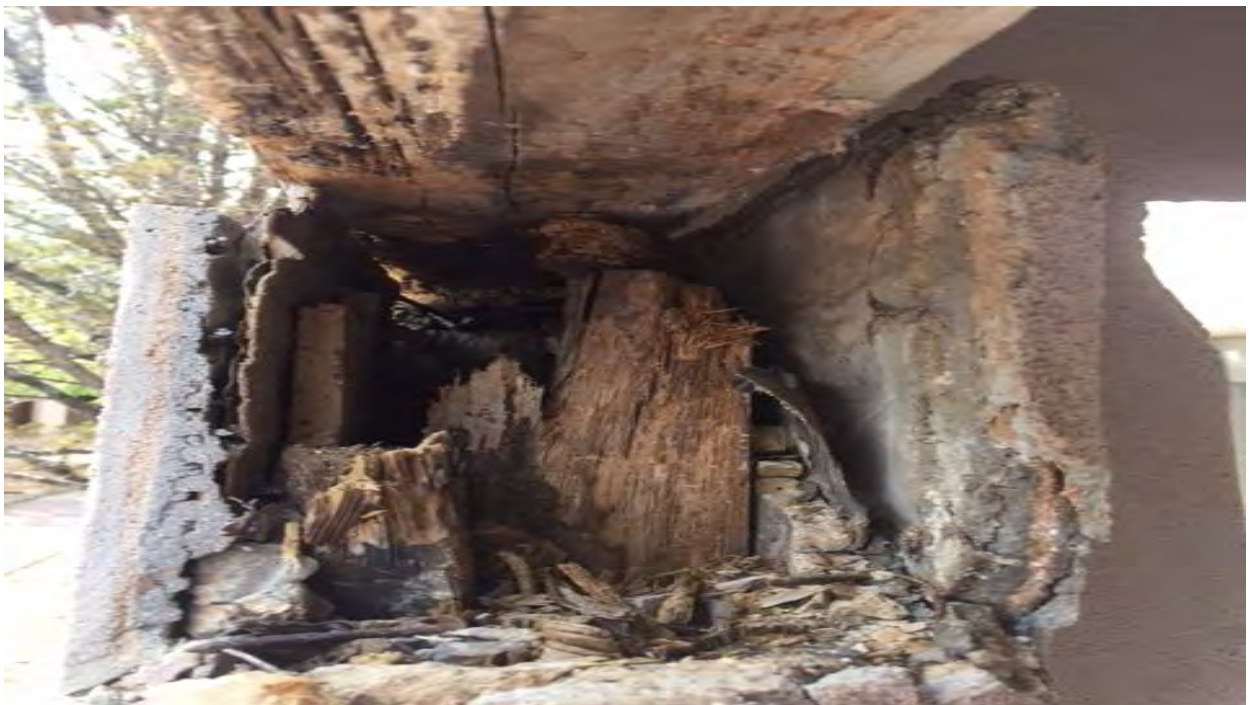
6. Header and Corbel water intrusion damage
