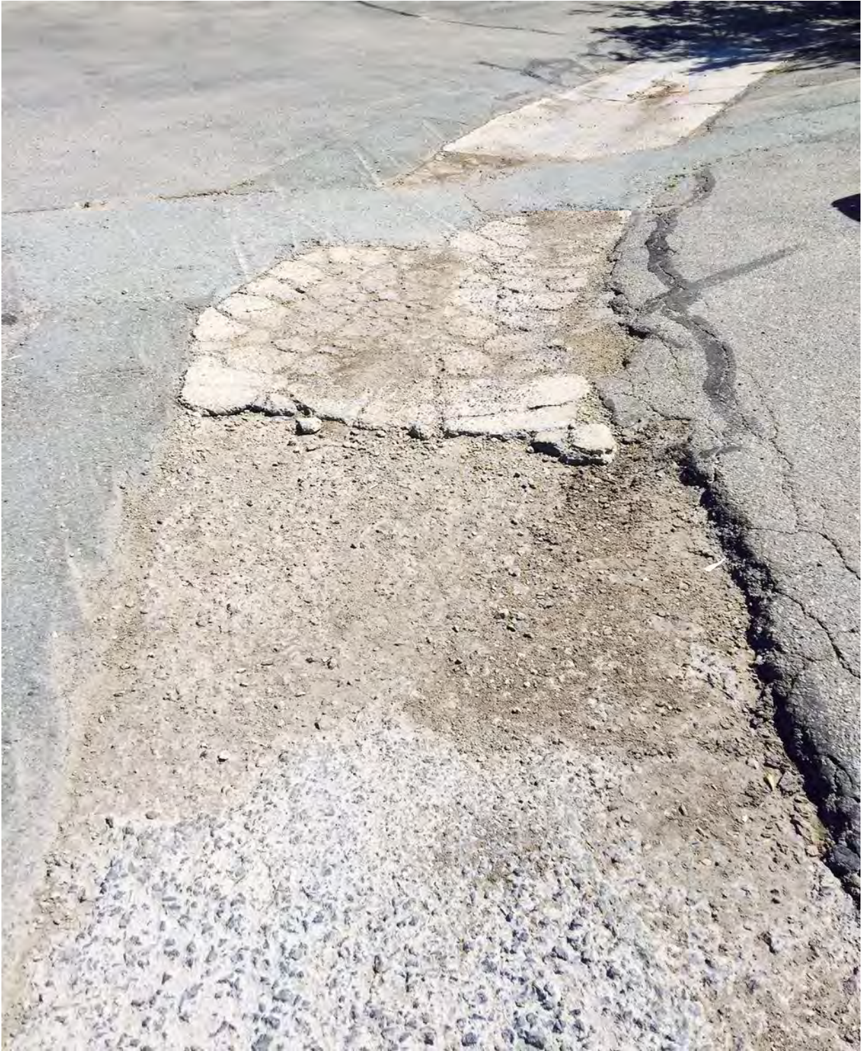
9. Parking lot weather and use deterioration
