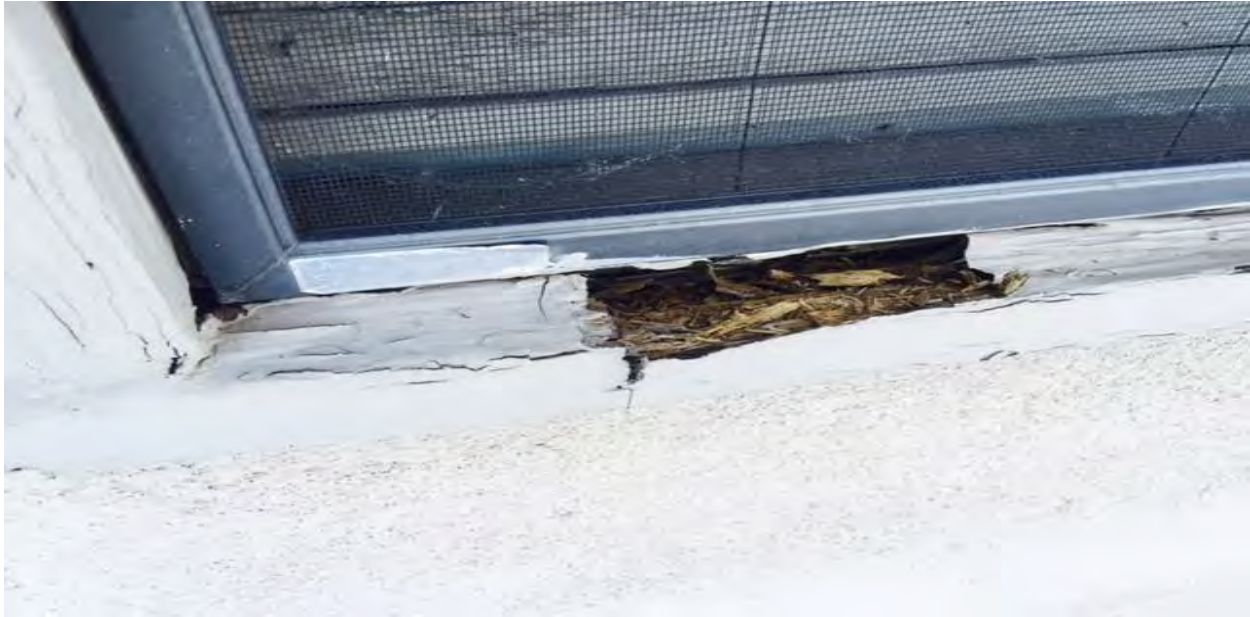
7. Window sill water intrusion damage
