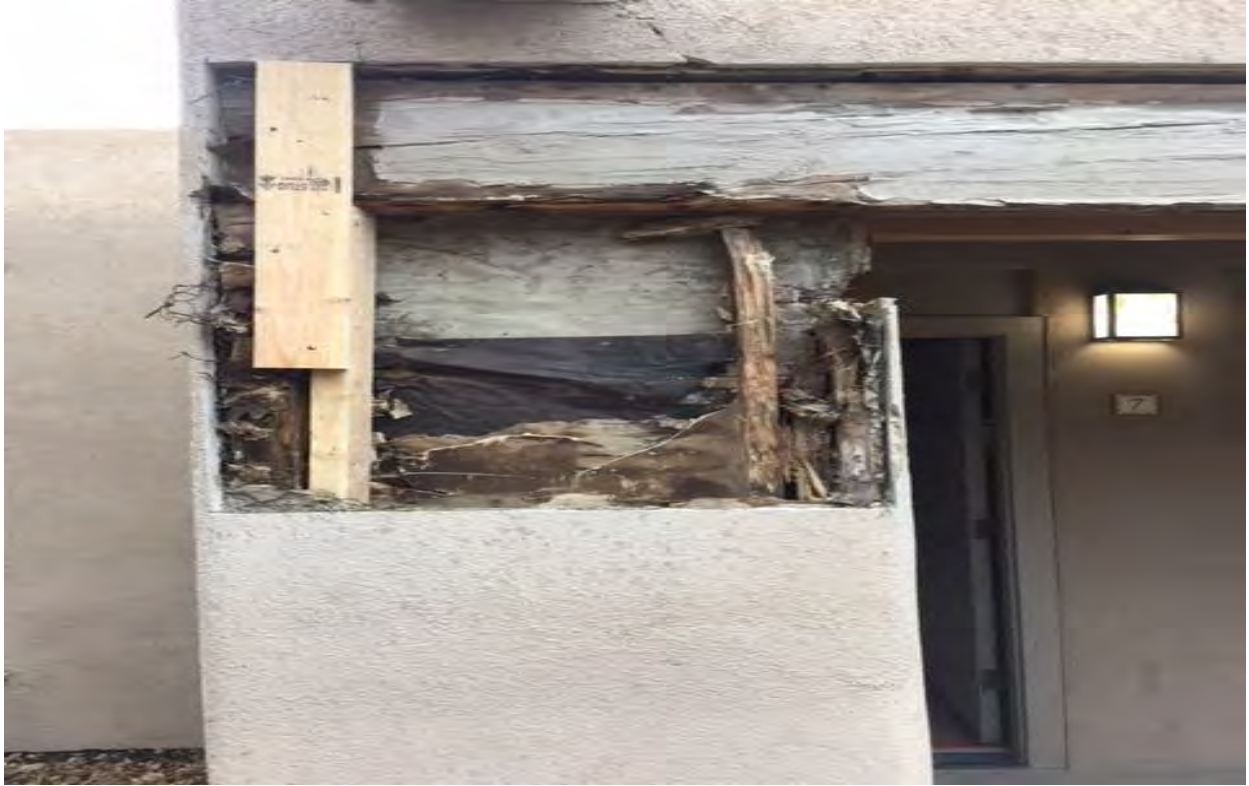
5. Header and Corbel water intrusion damage
