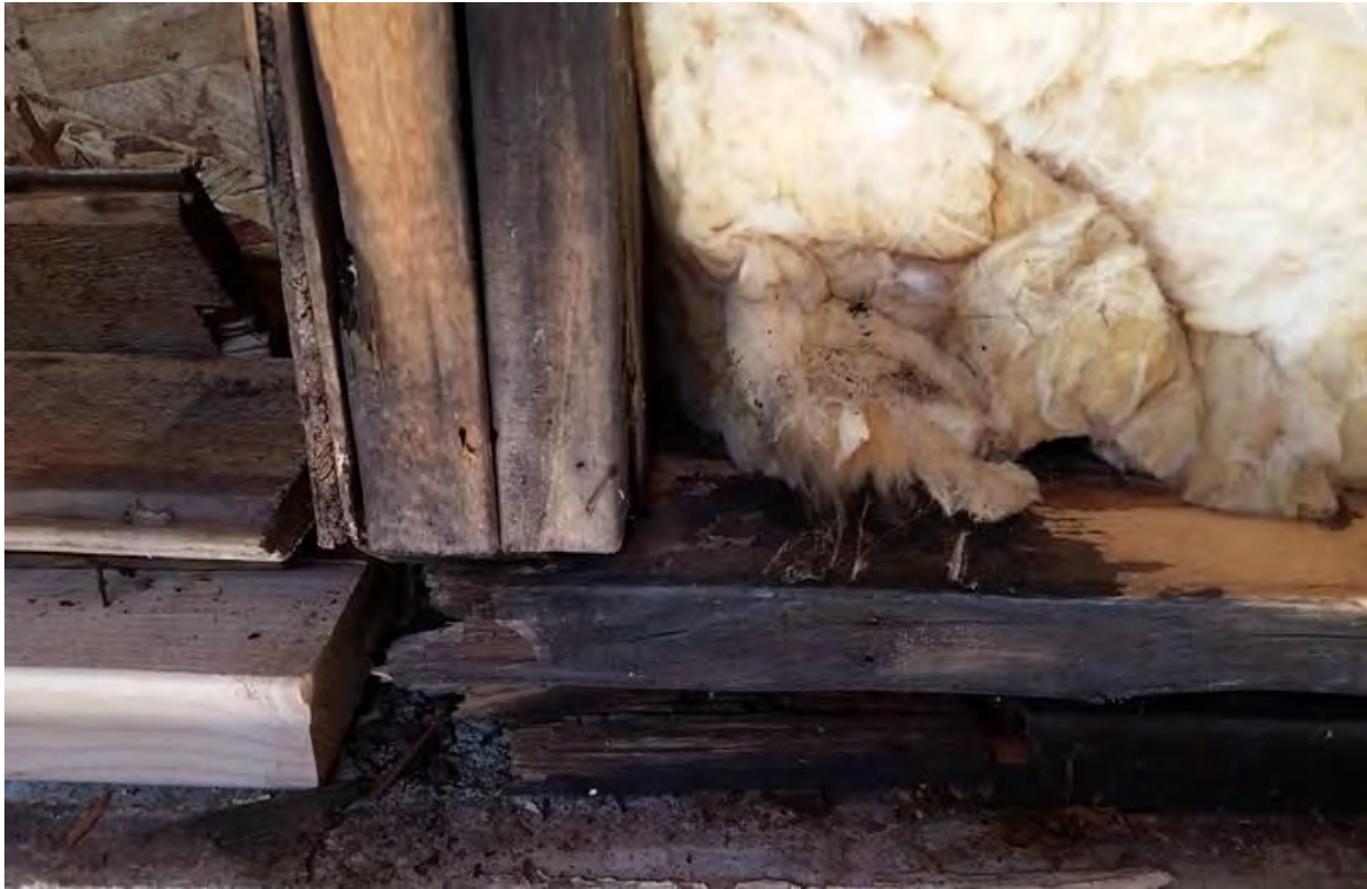
1. Pool facility exterior wall structural damage
