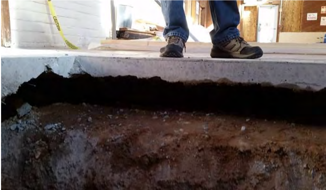
2. Pool facility foundation structural damage
